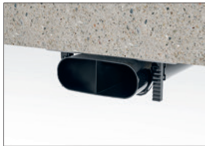
Shallow duct on the ceiling
